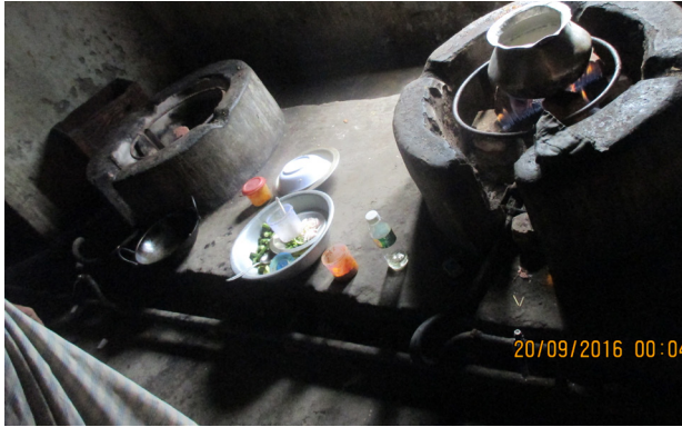
A burner being utilized inside the factory for cooking purposes. This is a dangerous practice and contrary to safety regulations, as it involves the use of open flames and non-compliant gas supplies.
