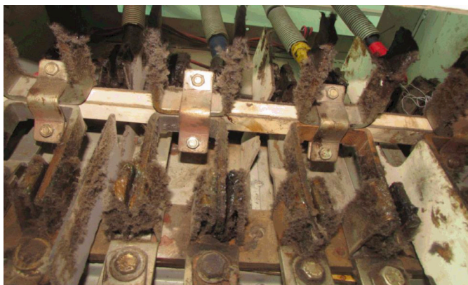
Dust and dirt accumulated on electrical wiring, which can cause sparks and start a fire. This fire hazard was identified at over 60% of the Accord-covered factories.
